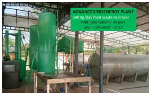
Large capacity (500 kg/day) food waste biogas plant installed at Trivandrum International airport.
