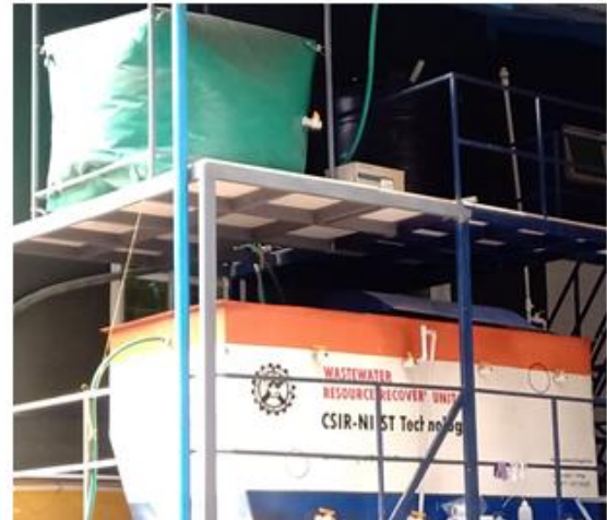
3 KLD unit treating Bakery wastewater
