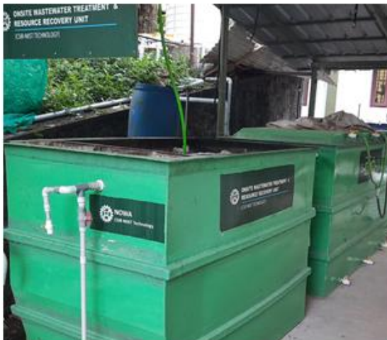
10 KLD unit treating canteen wastewater
